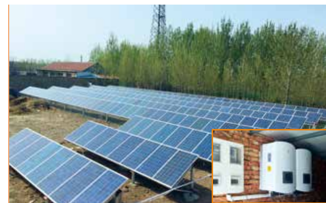
Shandong Leling poverty alleviation PV Plant 50kW
