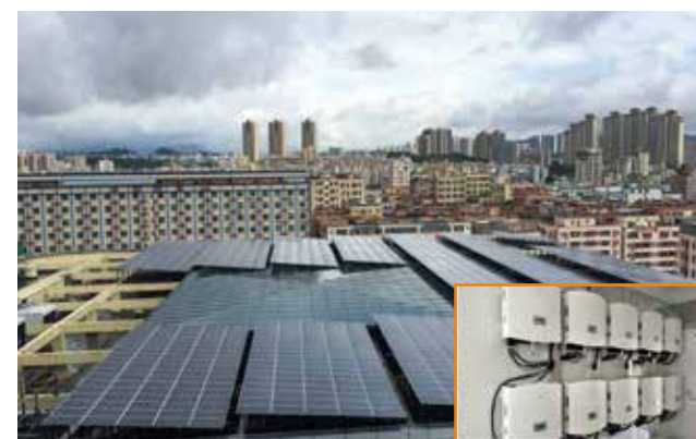
Shenzhen Jiangnan Times Building 600kW
