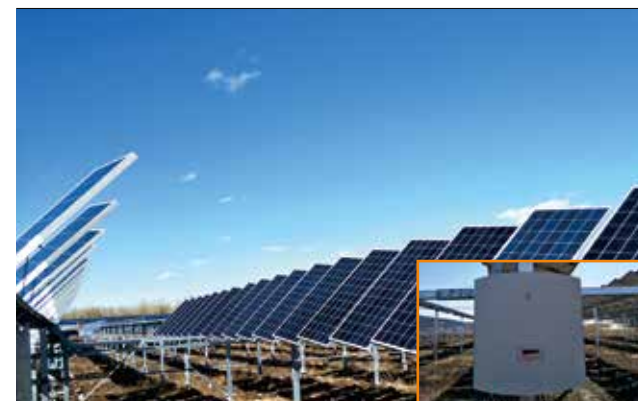
Hebei Zhangbei Agricultural-photovoltaic hybrid PV plant 50MW
