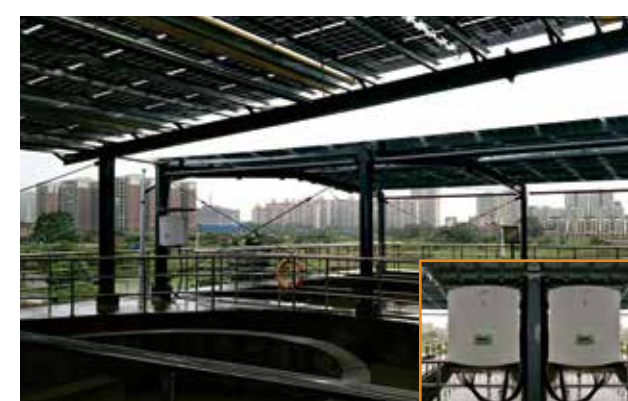
Hunan Yongzhou dao county water plant 800kW
