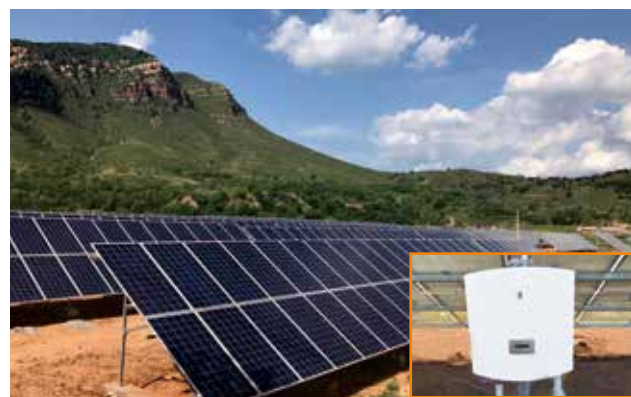
Shanxi Xiyang poverty alleviation PV Plant 7.2MW
