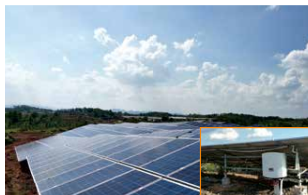
Jiangxi Ganzhou PV Plant 3.5MW
