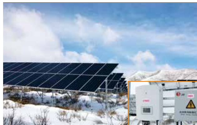
Shanxi Guangling PV plant 1.47MW
