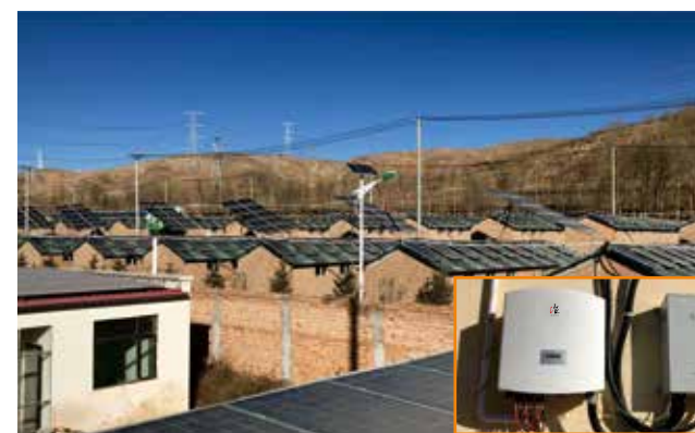
Qinghai HuzhuBanyan poverty alleviation PV Plant 2MW
