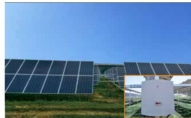
Hebei Zhangjiakou poverty alleviation PV Plant 5.1MW
