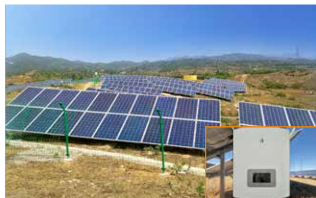
Hebei Qinghuangdao poverty alleviation PV Plant 9.7MW
