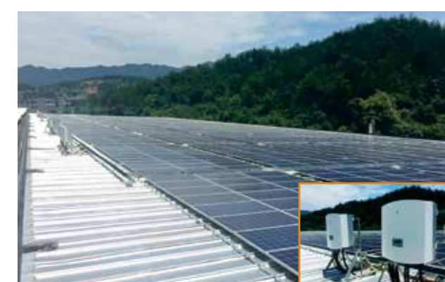
Hainan JiuLongGlass 1.7MW
