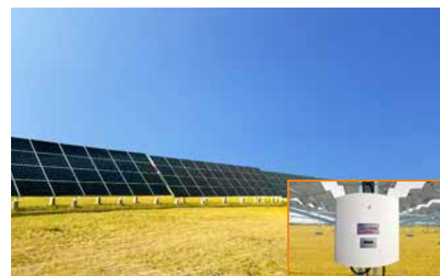
Huaneng Yimin surface mine PV plant 20MW
