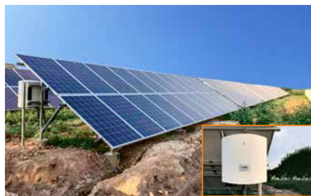
Hebei Qinghuangdao poverty alleviation PV Plant 5MW
