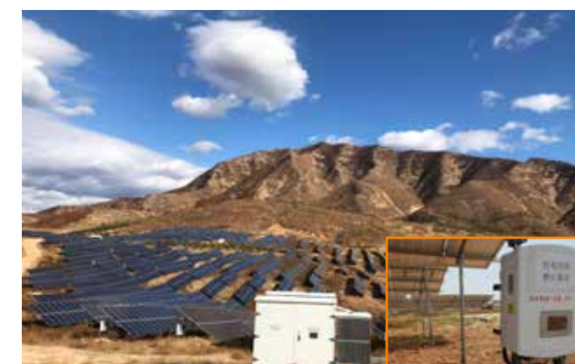
Liaoning Gaizhou Jiuzhai PV plant 20MW
