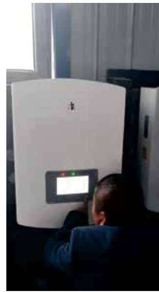
Heilongjiang PV plant
